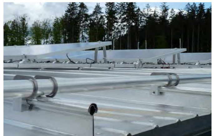
Snow guard on round bulb seam roof with RoofTech Single Tube Holder Type B on S-5!® Z-Mini clamp. Very stable and discreet .
